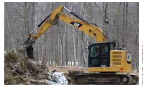
An excavating crew from Atlantic Landscaping Construction works to transform a former septic field at Sieur de Monts Springs into a forested wetland.
