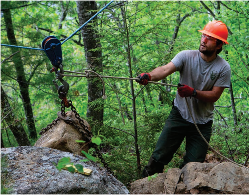
Acadia National Park trail crew member Max Wither works to ease a boulder into place while replacing part of Kurt Diederich's Climb on Dorr Mountain in Acadia National Park.
