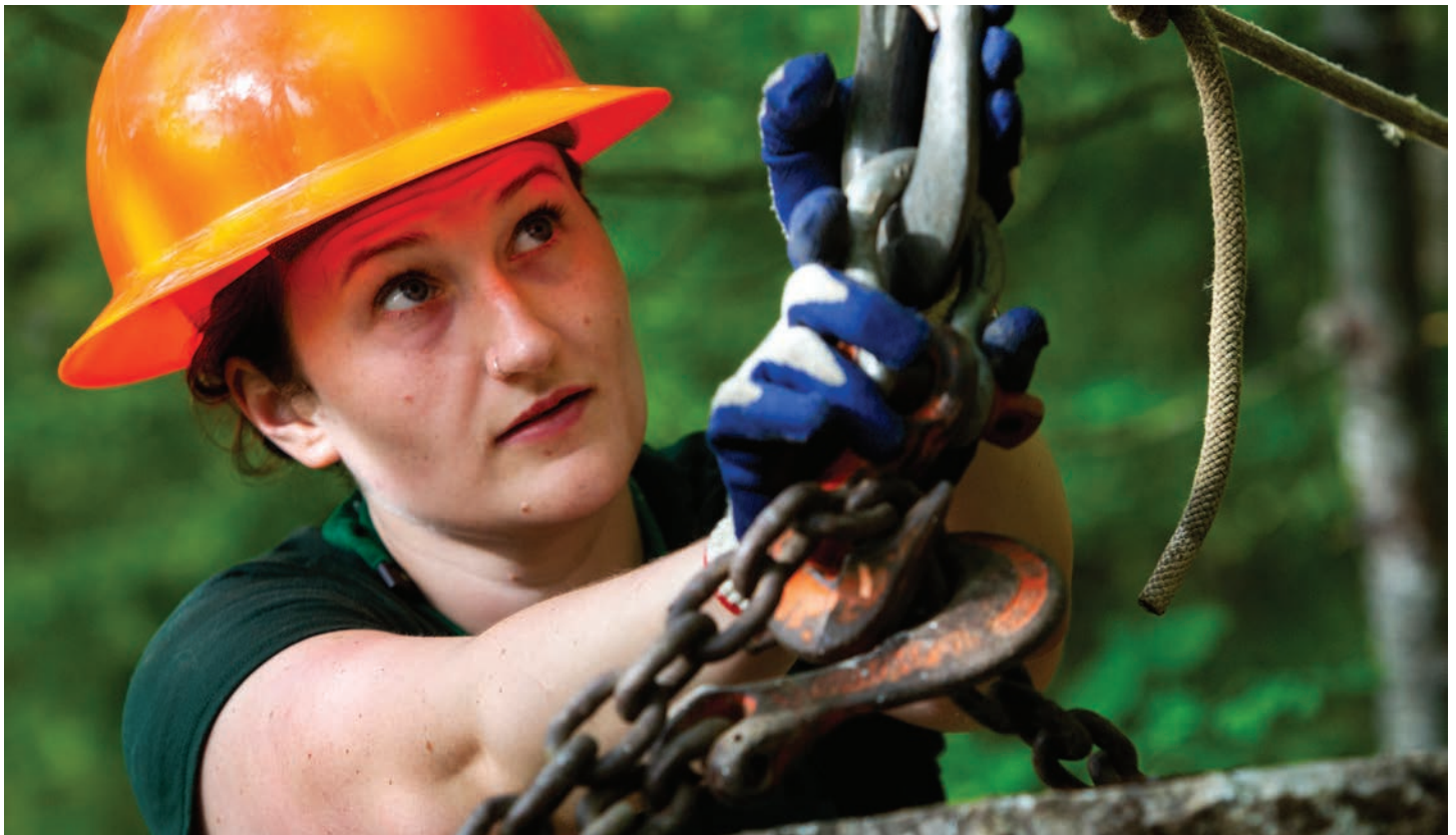
Acadia National Park trail crew member Isabella Connelly adjusts chains used to maneuver a rock into position while working to repair Kurt Diederich's Climb on Dorr Mountain in Acadia National Park.
