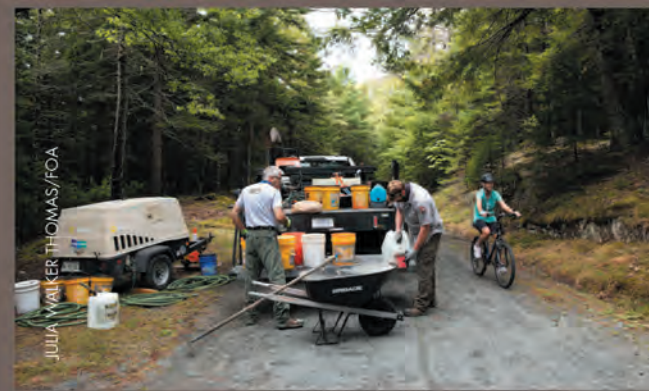
BELOW: Master Mason Mike Fitzpatrick and Mason Helper Ryan Meddaugh mix mortar on-site at the Amphitheater Bridge. BELOW BOTTOM: Mason Helper Ryan Meddaugh pressure washes lichen off the stone. Lichen degrades the structure of stone, and over time can cause it to crumble.
