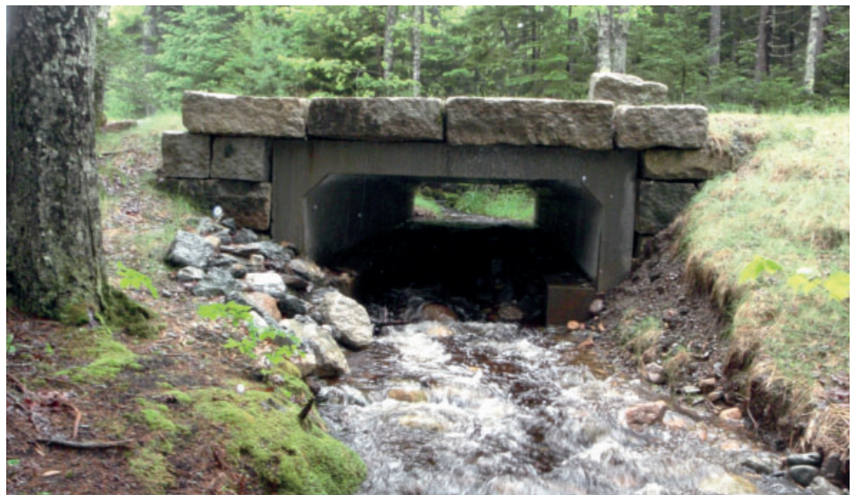
Culvert replacement on the Stanley Brook tributary off Wildwood Stables Road. Before restoration (top), the corrugated metal culvert is perched above the stream and poses a barrier to fish passage. After restoration (bottom), the concrete open-box culvert allows unimpeded fish movement and accommodates greater stormwater flow.
