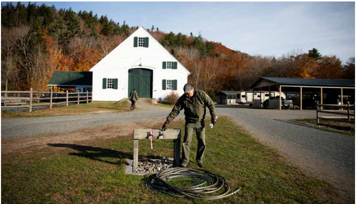
Acadia National Park plumber Jeff Chamberlain works on draining a seasonal water line at Wildwood Stables to prevent damage from the winter freeze-up.
