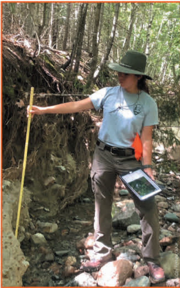
Acadia's Physical Science Technician Erica Doody measures the depth of scour that occurred to a section of Chasm Brook.
